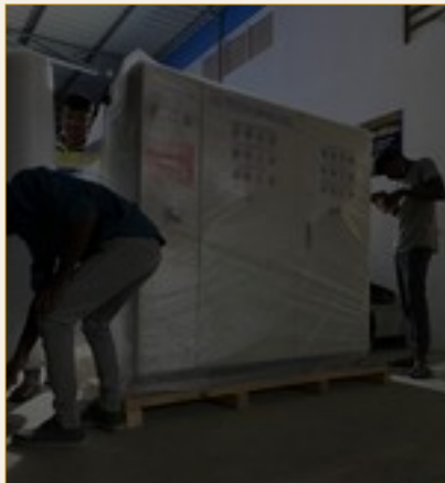
ELECTRICAL PANELS SECTOR 07
